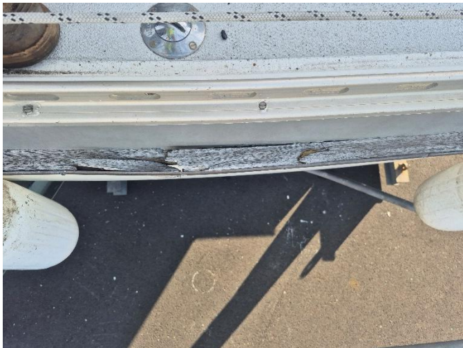
Damaged rubbing band
